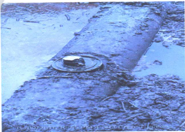
Figure 1: Cut-off cone on the pipeline.
